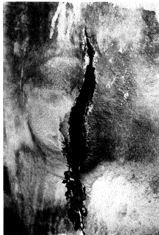
Figure 3. Vertical crack in the water jacket.
